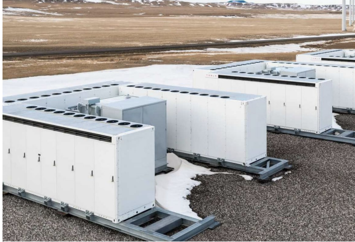
Stationary Energy Storage
